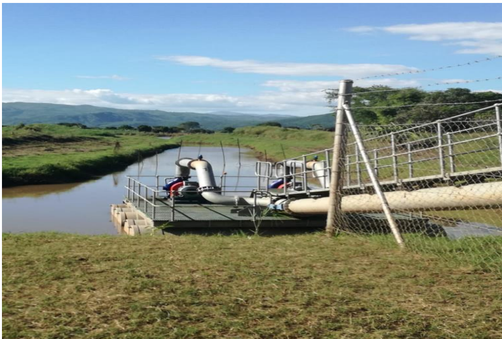
Figure 3: Phata Water Intake Point
